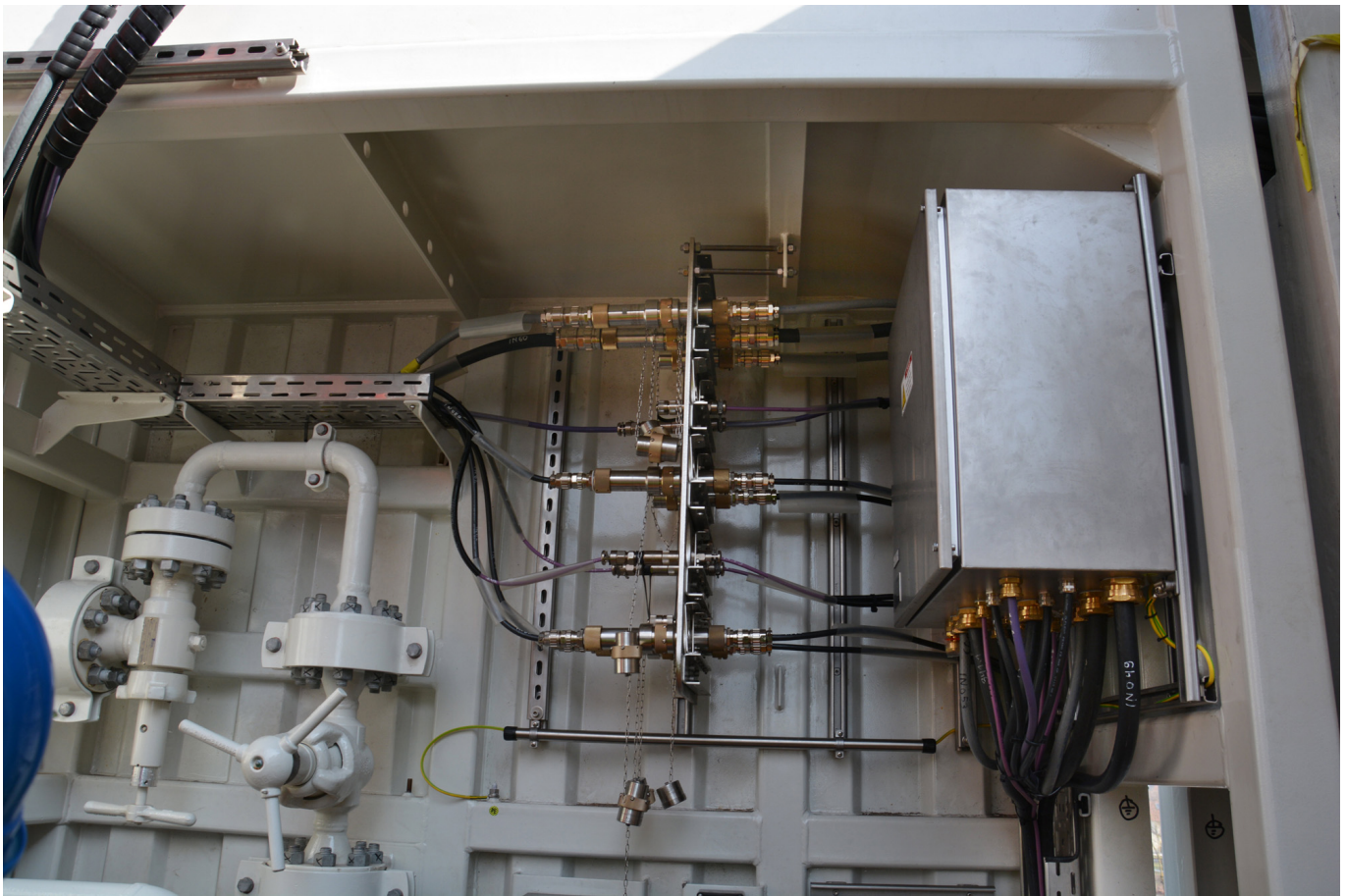
Fig. 3: HAWKE connectors (l) and HAWKE cable glands (r) in use –created for tough and potentially explosive environments. (Photo: Jacob)
